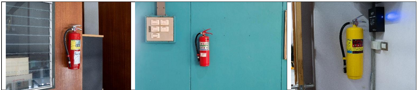
Fire Extinguisher (Songkhla Rajabhat University)
