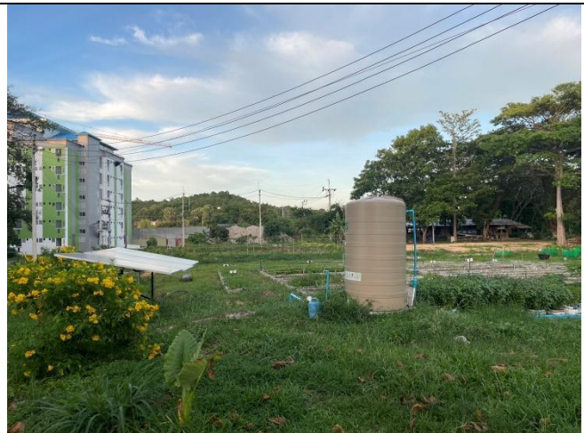
Water storage tank and pipe distribution system used to store and distribute non-potable reused water for plant watering and landscape maintenance.
