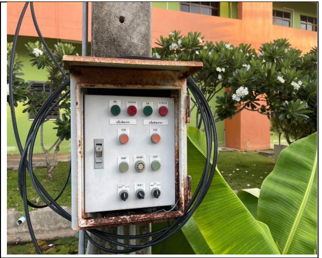
Aeration control panel used to operate aerator units for improving the quality of treated water in the campus pond system.
