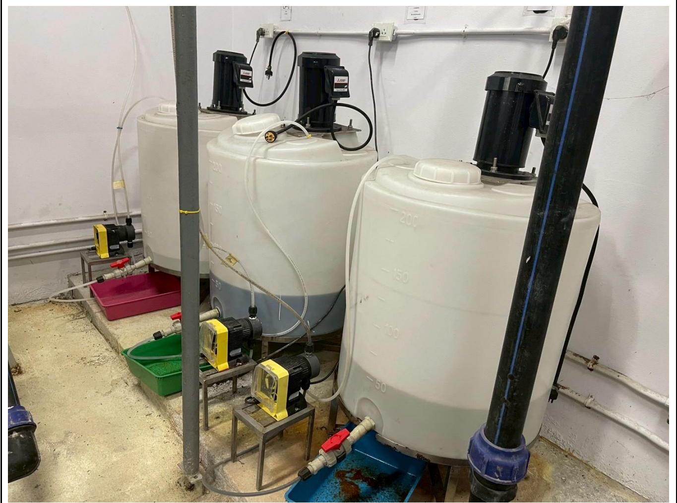
A wastewater conditioning and disinfection tank used to adjust and disinfect treated wastewater before discharge into public waterways.
