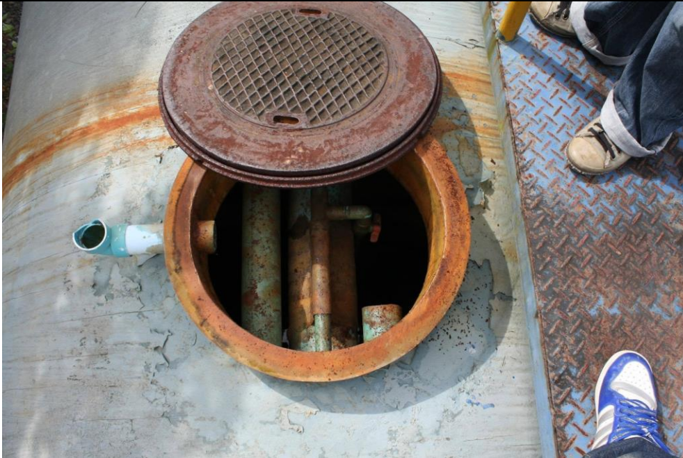
monitoring wastewater treatment plant at Songkhla Rajabhat University
